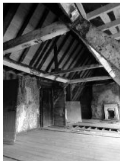
Above, Architectural conservation site, Number 9/9a Aungier Street, Dublin, Ireland. Courtesy Sunni Goodson and McGrath Group
